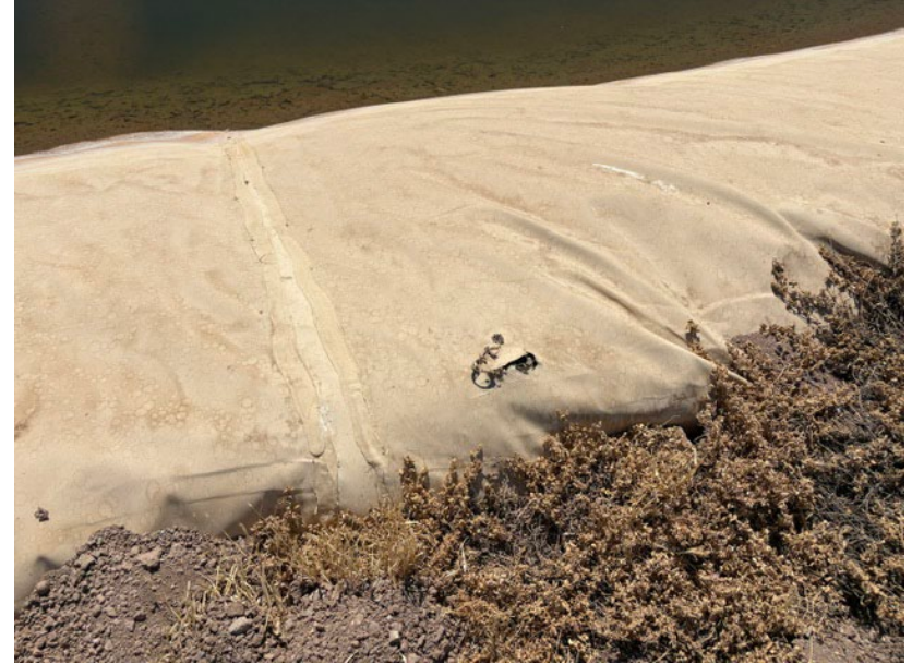
Raw Water Pond no. 2 – lining has deteriorated and the District is losing water to percolation
